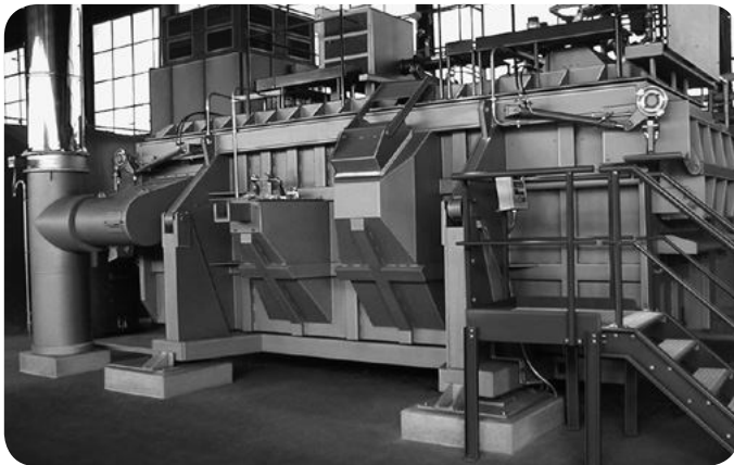
Aluminium industry: smelting furnace
