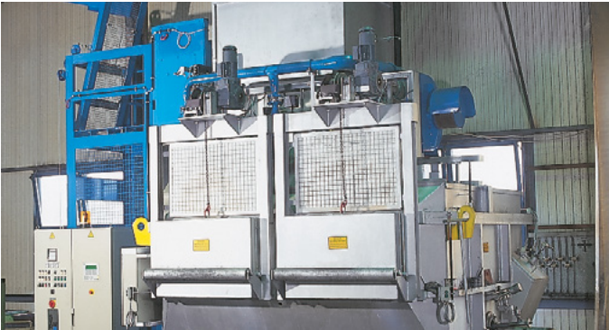
Aluminium industry: shaft melting furnace
