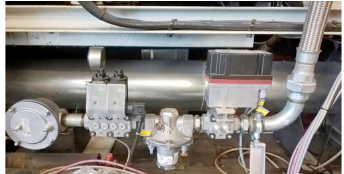
CHP for generating electricity and heat
